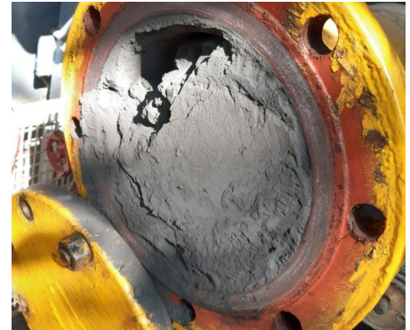
Black Powder accumulated in gas transmission pipeline. Image courtesy of ROSEN Group
