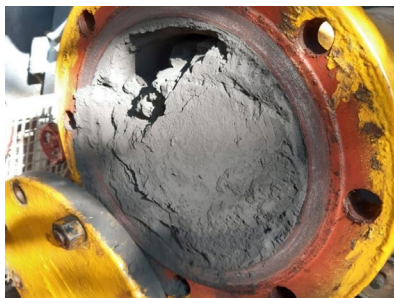
Black Powder accumulated in gas transmission pipeline. Image courtesy of ROSEN Group
