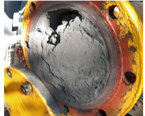
Black Powder accumulated in gas transmission pipeline. Image courtesy of ROSEN Group
